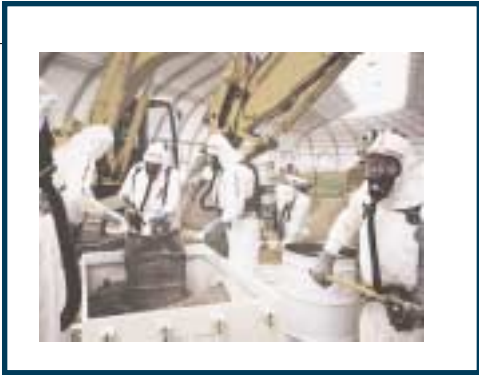
Effective cleanup of the Site requires a thorough understanding of how actinides move in the environment.
