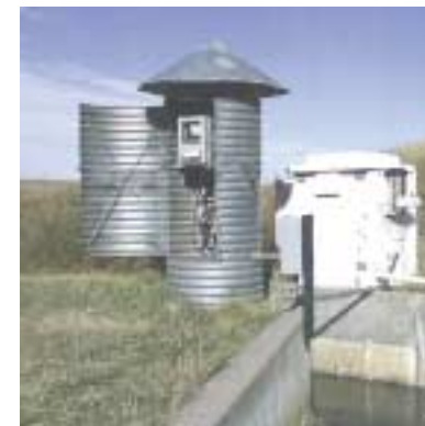
Surface water is monitored throughout the Site at automated stations. When the water flow rate of the water increases, this unit is programmed to increase the number of samples it collects.
