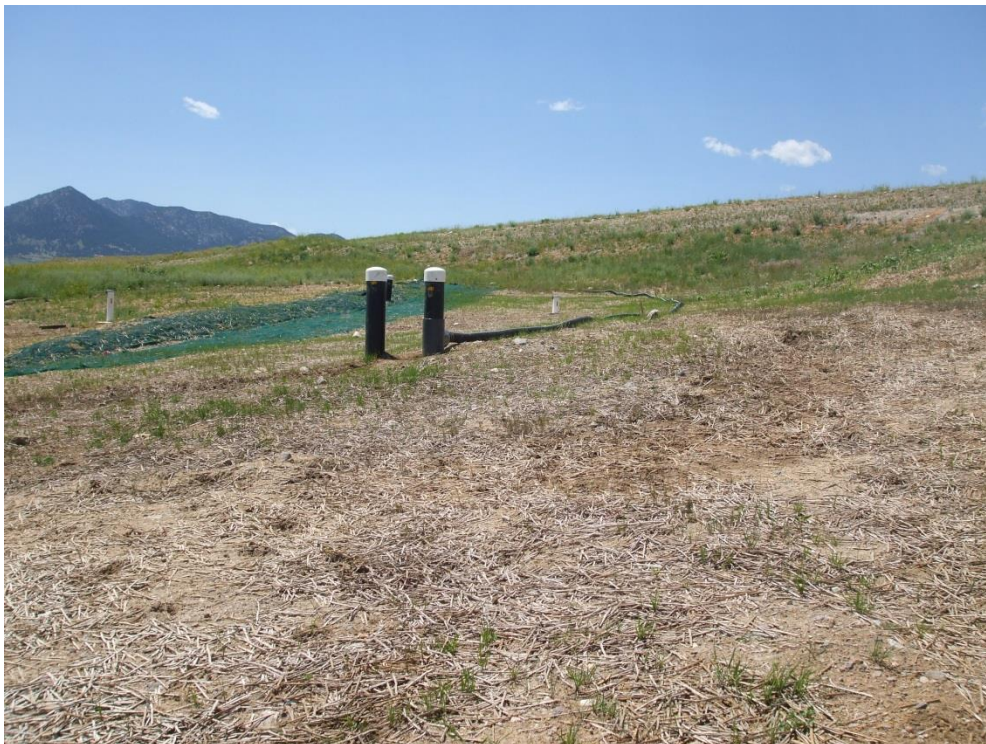
Figure 8: Looking West, the Gravity Drain Line from the Groundwater Intercept Wells Is in Place and Connected to the Flow-Through Line Installed in the East Subsurface Drain
