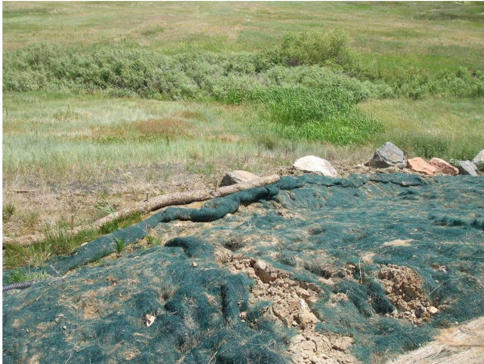
Figure 7: Looking Southwest at the Wet Area Created by Movement of the Toe of the Slump into the EPC
