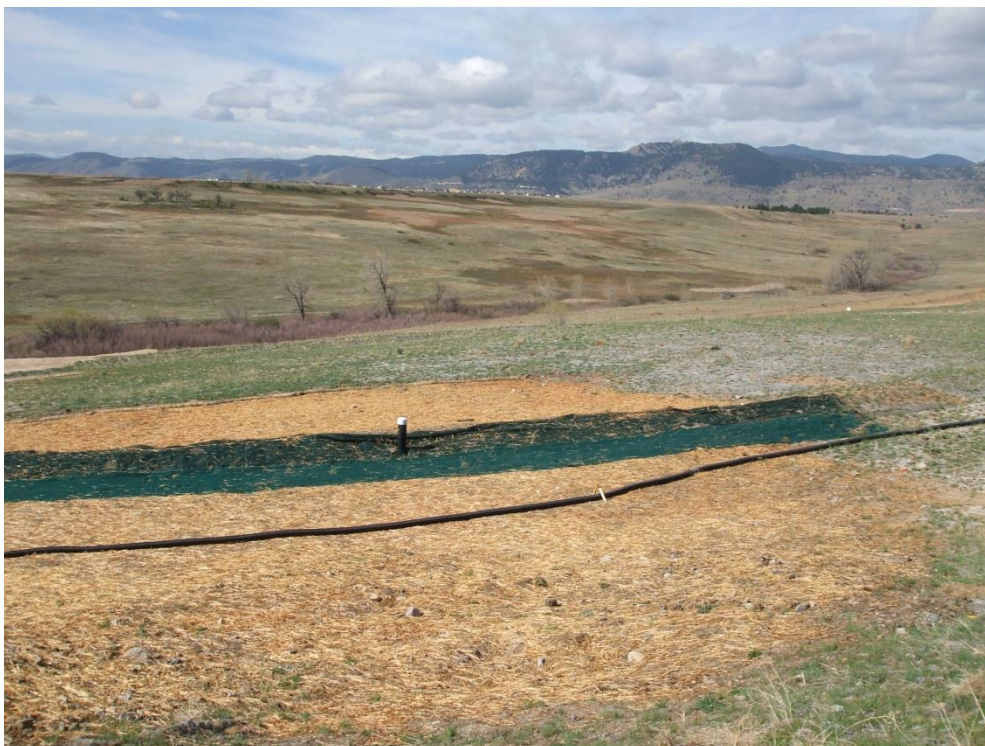
Figure 2: Looking South towards Berm 4 at the Aboveground Drain Pipe Running from the OLF GWIS to the ESSD and the 2015 OLF Grading and Berm Repair Location
