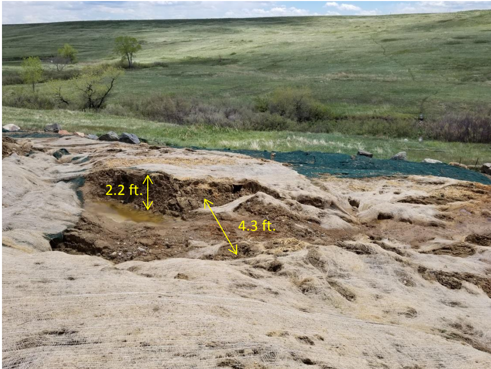
Figure 3: Standing on Berm 7 Looking Southeast at the Slump Movement. The scarps range from a few inches on the sides to 2.2 feet toward the center. The crack pictured above is one of the largest at 4.3 feet in width.
