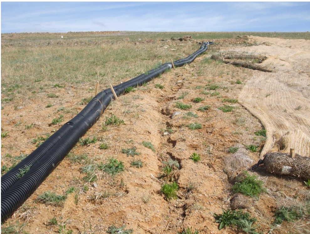
Figure 6: Standing Between Berm 7 and the EPC Outfall, Looking North at the Discovered Gully
