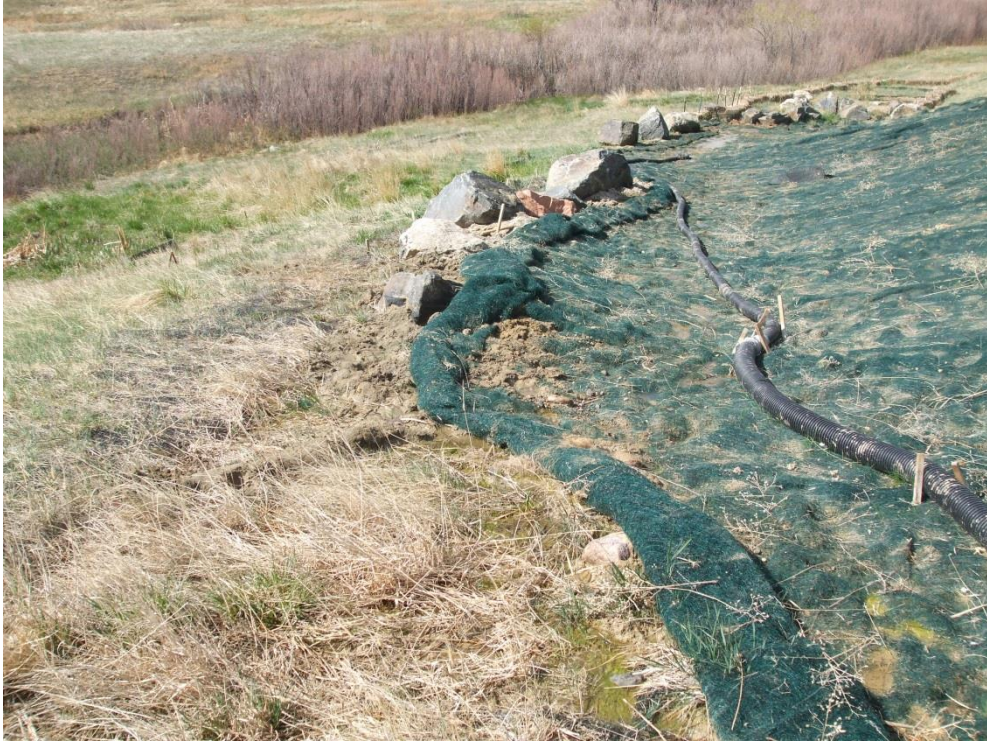
Figure 7: Looking Southwest at the Area that Is Contributing to the Wet Area Located South of the EPC Side Slope Bank
