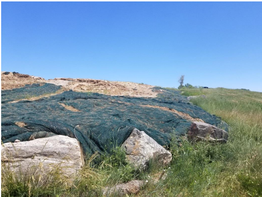
Figure 6: Looking North at the Area of the EPC Outfall That Is Blocked by the Recent Slump
