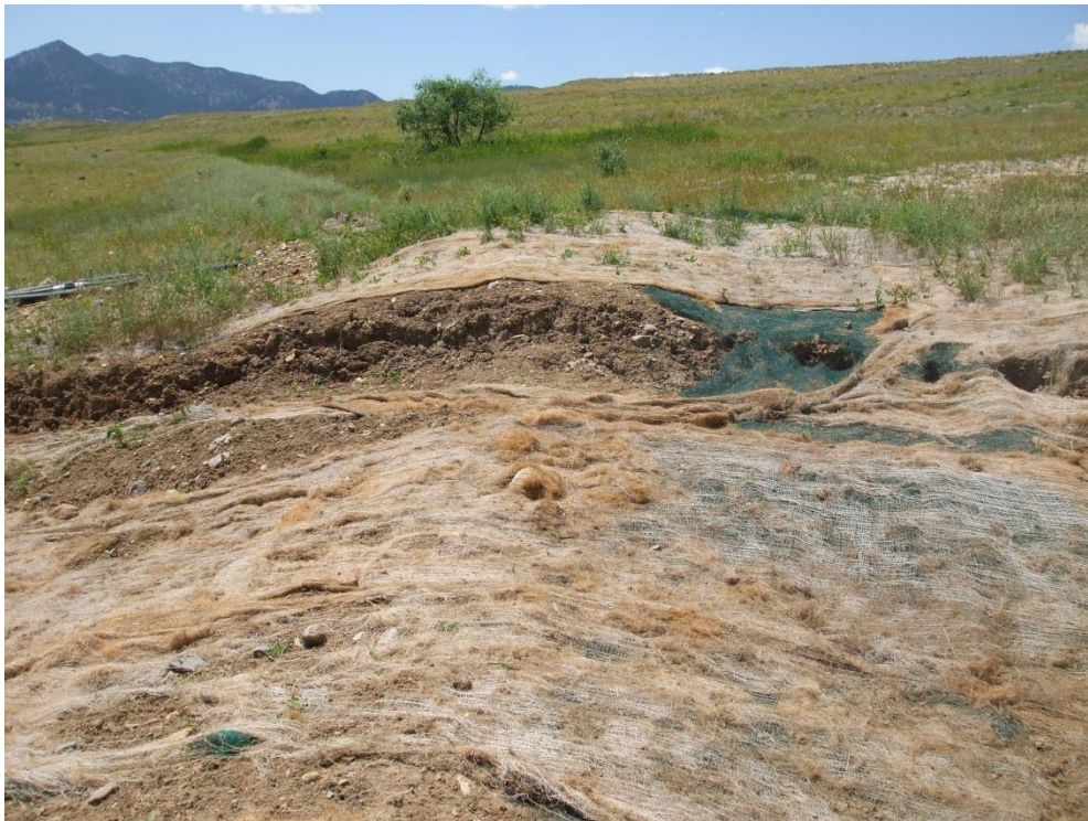
Figure 4: Looking West at the Depth (10–12 inches) of the Crack That Runs North and South Through Berm 6 and 7
