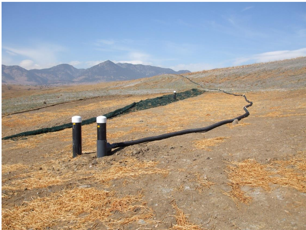
Figure 4: Looking West at Berm 4 and the Gravity Drain Line Connection to the ESSD Pictured as the Black Risers
