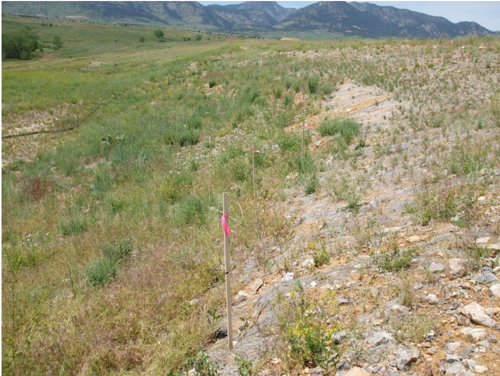
Figure 5: Looking West at the Staked Crack Above Berm 4
