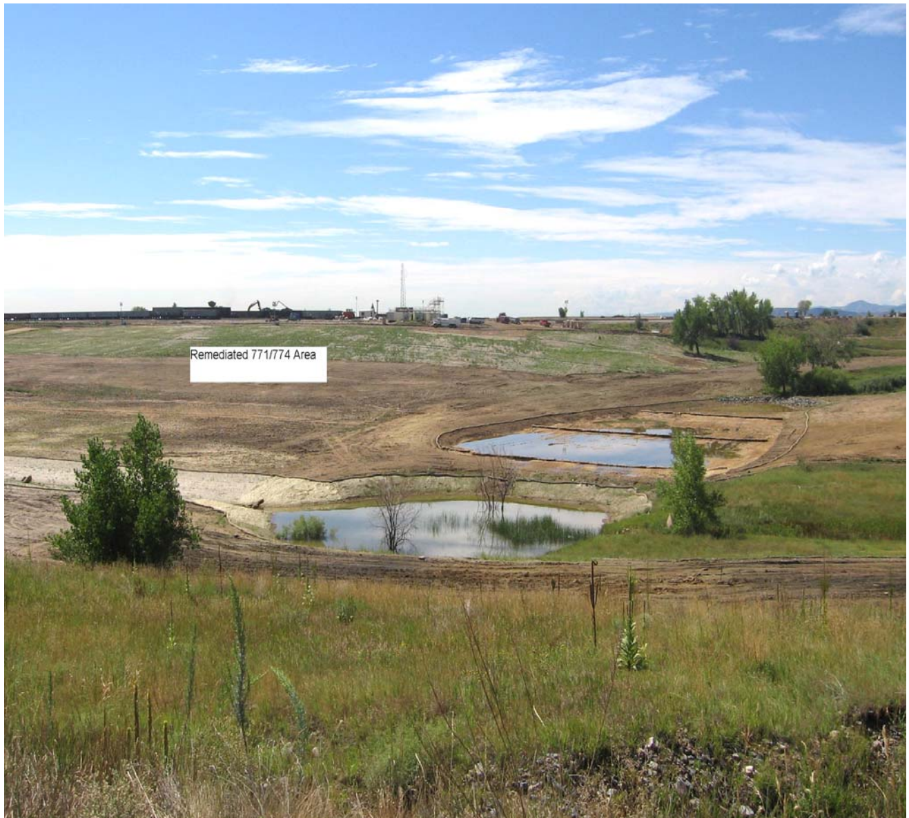
Figure 4. View looking south from August 2005 showing completed remediation of 771/774 at approximately the same location as Figure 3. Note: new wetlands have been added to the area and at the top of the slope one can see railroad cars being loaded with low level radioactive debris waste from the demolition of B776/777. These specialized railroad cars will carry the debris waste to the low-level radioactive waste disposal site, Envirocare of Utah.
