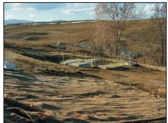
The newly installed vault is visible between the cells at the completion of the media replacement project.
