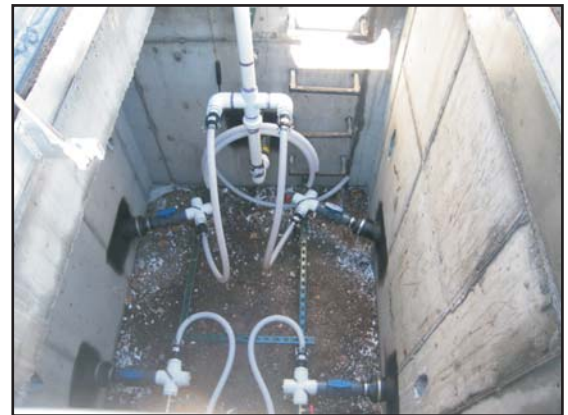
A feature of the new vault installed as part of the system improvements is that the plumbing configuration can be easily changed and new pipe liners installed.
